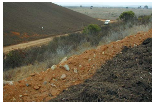
San Diego's Greenery supplied mulch for this California Department of Transportation erosion control project, where the product was applied to a freshly graded hillside.
