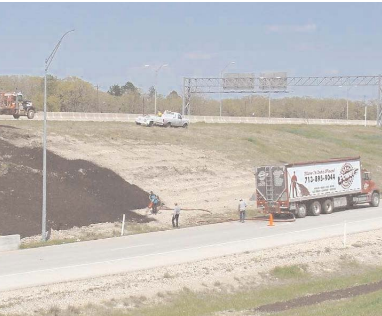
A pneumatic blower truck is used to ease application of an erosion control mix on a roadside slope in Texas.
