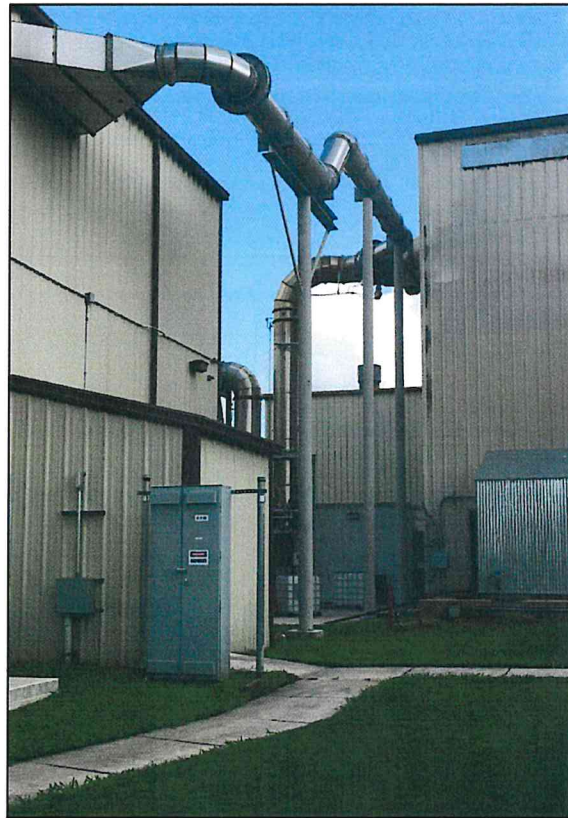
Figure 5. Photographs of the supplementary ductwork, dampers, and valves.
