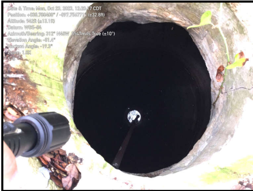
S-8: Note the water line inside the cistern.
