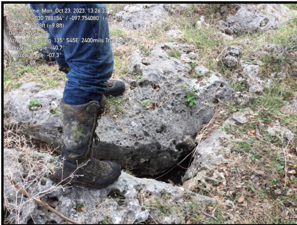
S-9: Solution cavity located on the southcentral part of the Site.
